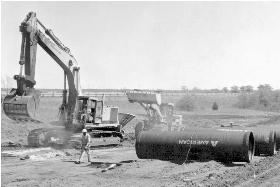
60" AMERICAN Fastite® Joint Ductile Iron pipe being installed as a water transmission main.
